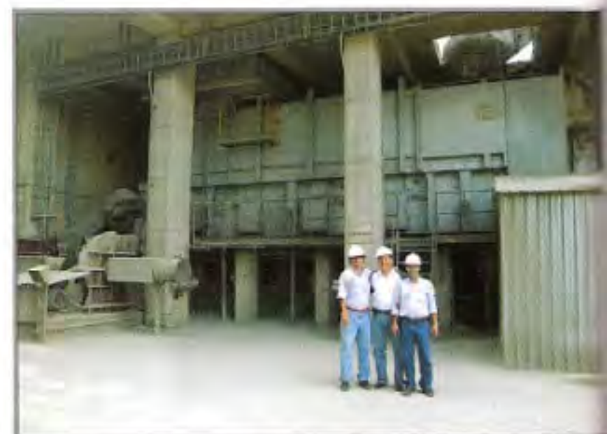
出口巴西的篦冷机运行良好 Grate cooler exported to Brazil
